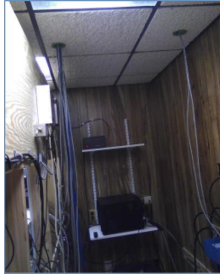
Suspended ceiling "grommets" provide out-of-sight, out-of-the-way, overhead cable-paths for rotor, RX antenna & Stack Match control cables.
