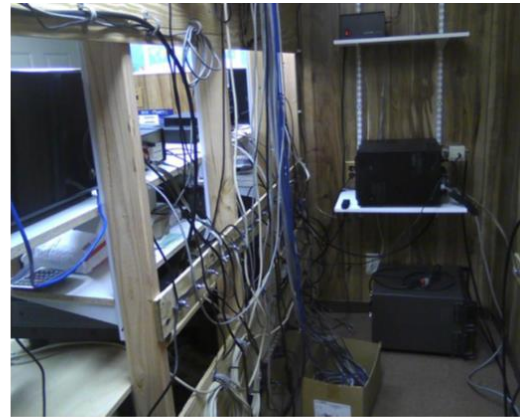
Here's what wiring looks like in a 42" workspace. Note the spare IC-4KL amp on the floor below the PW-1.
