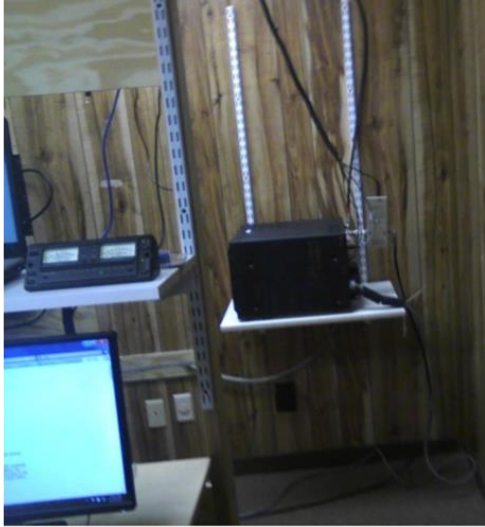
A pair of PW-1 KW auto-tuned amps is shelf-mounted, out of operational view, in the technical workspace behind operating desk.
